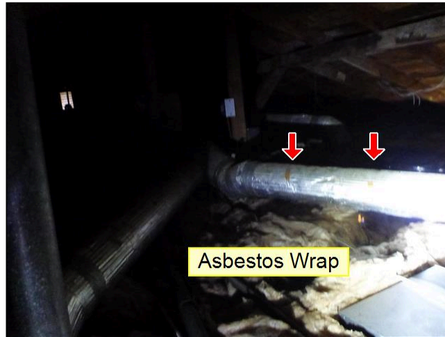
10.6 DISTRIBUTION SYSTEM (See Picture(s))
